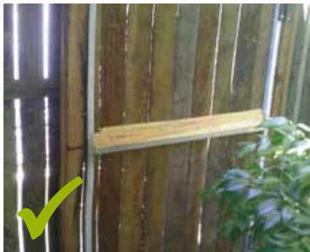
A minimum 60 degree angled wedge along the horizontal rail eliminates a foothold.
